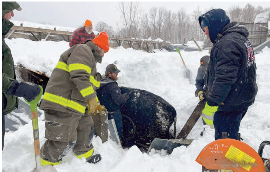
The Western Volunteer Fire Company in Oneida County helped rescue animals from the 100' x 300' barn after the roof collapsed at Sokoloff Farms, Booneville, claiming up to two-thirds of their herd. Photo provided
